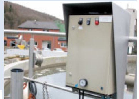
Sewage treatment plants Oxygen measurement in an aeration tank – a Rittal KS enclosure protects the sensitive electronics.
