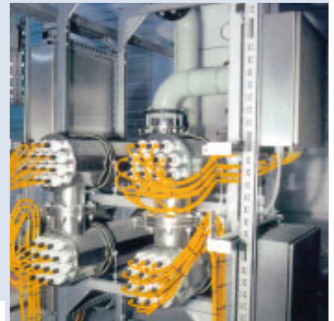
Drinking water processing Rittal compact enclosures from the AE series (stainless steel) are used, for example, in a drinking water processing plant with UV radiation.
