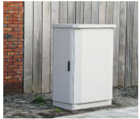
FTTC – enclosures with concealed climate control with no visible vent slots.
